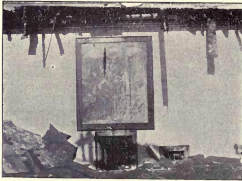
COURT ROOM AFTER THE FIRE.
